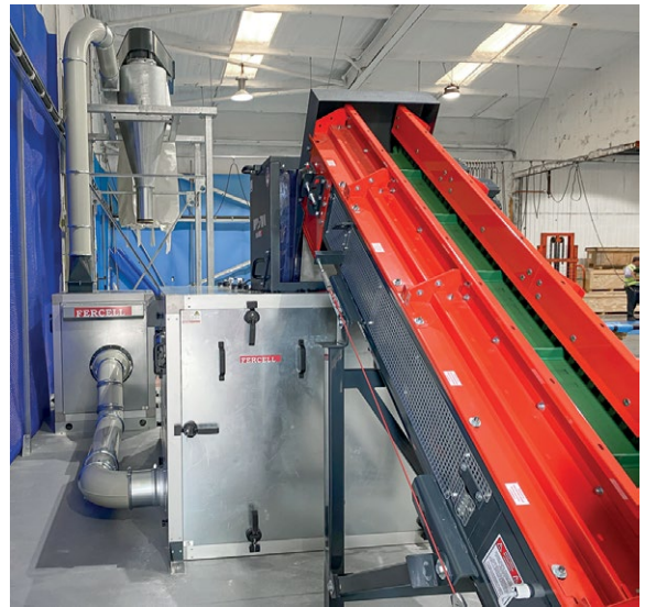
Conveyor technology between the pre-shredding and post-shredding of WEIMA
